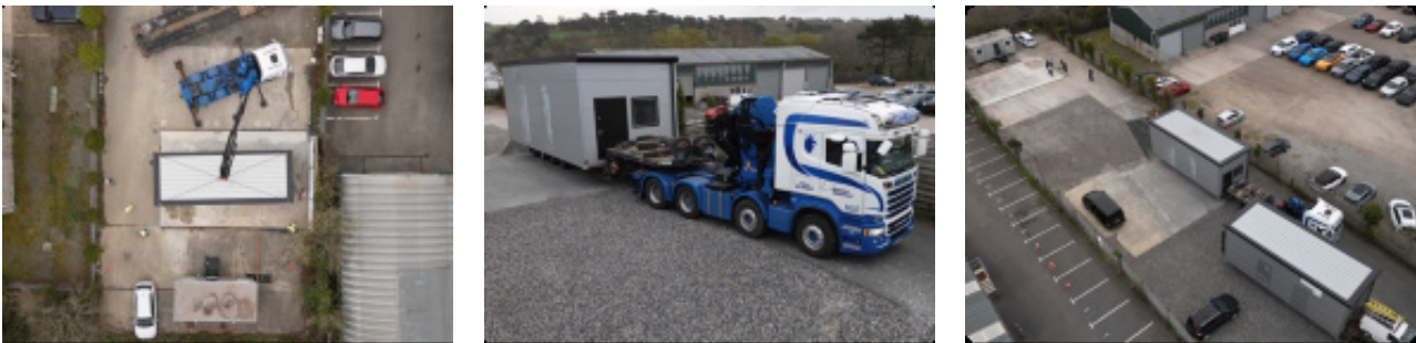
Figure 10: Installation of Revolution-ZERO reprocessing unit for Royal Cornwall NHS Hospitals Trust (Cornwall NHS)
